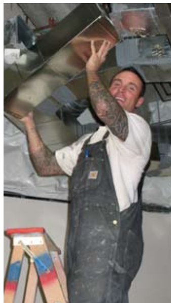
Payton Perkins from Apollo Sheet Metal installs metal ducting. This ducting will help create a sterile environment for surgery by directing clean air down to the surgical table and producing a curtain of air to surround the patient and surgeons.
